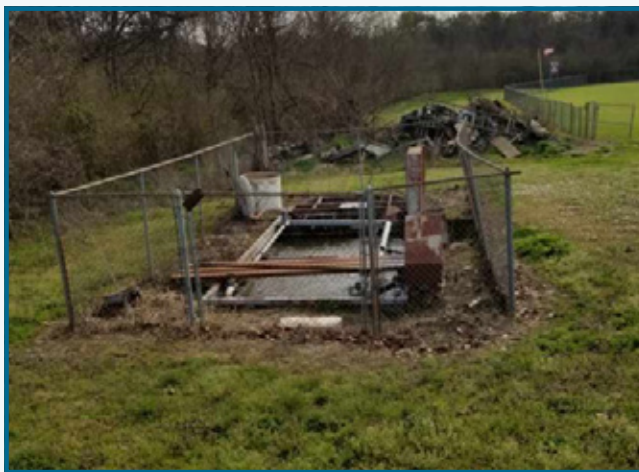
Photo courtesy of Forest High School Current conditions at the wastewater treatment plant at Forest High will soon change thanks to upgrades funded by the State Revolving Fund loan program.
