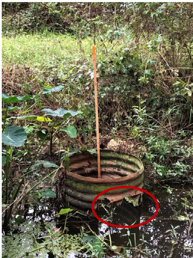
Figure 6 – Water level control structure with missing flap gate at northeast corner of the effluent distribution area
