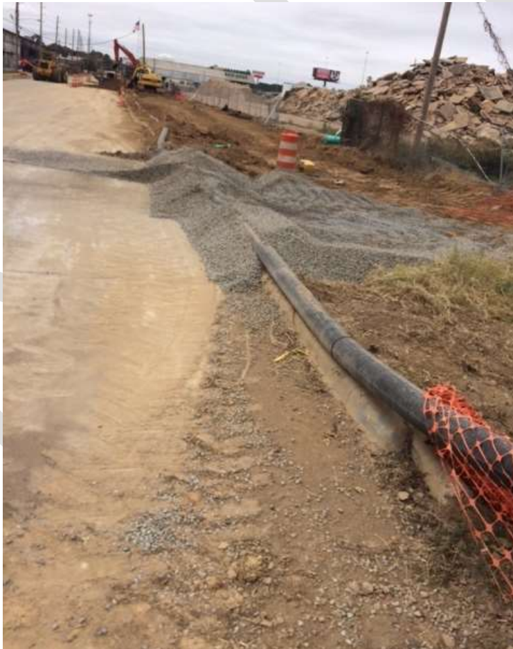
Picture 5: Bypass piping for lift station rehab project
