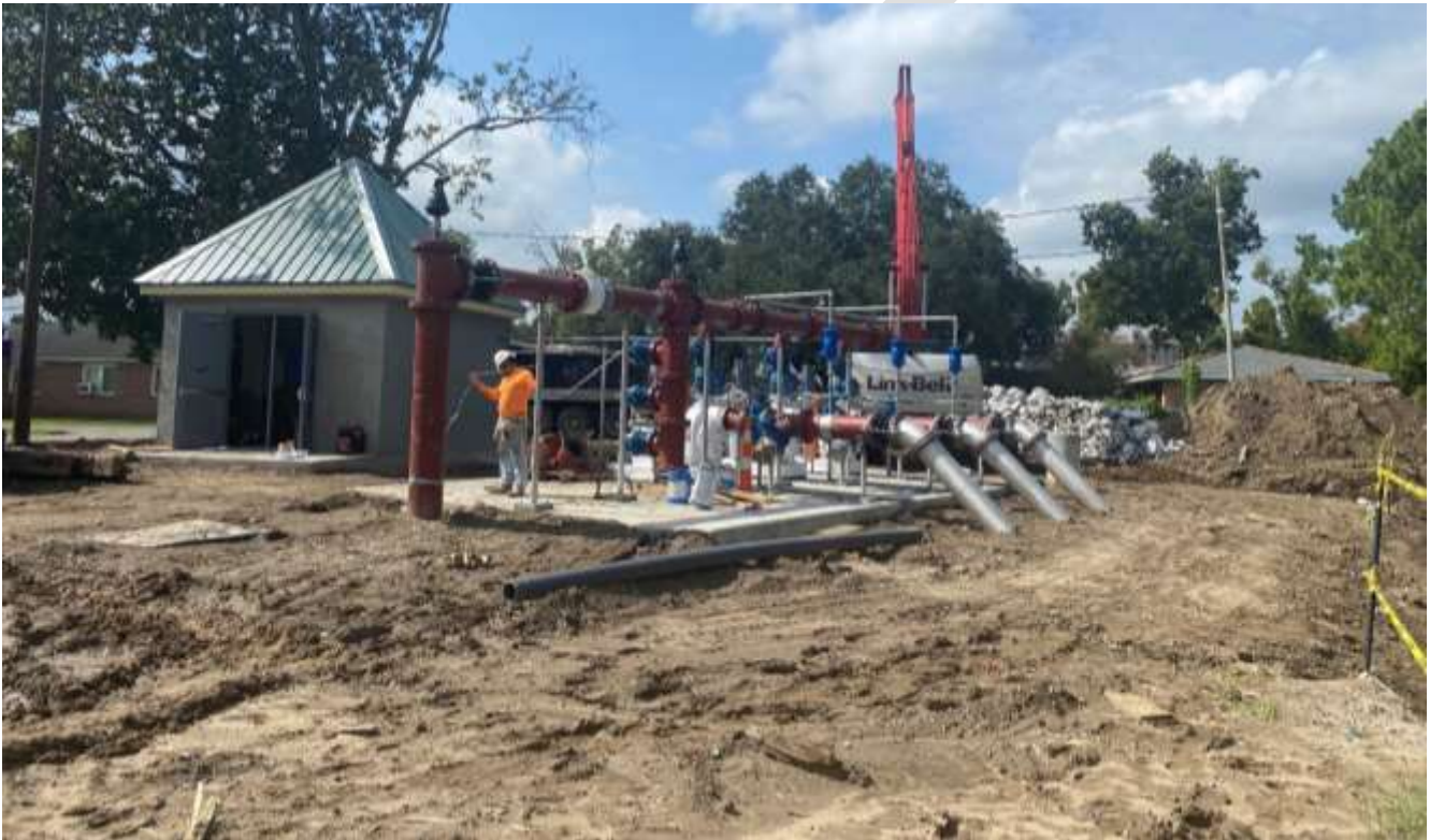
Picture 4: Water intake manifold for BLFWD {320 project}
