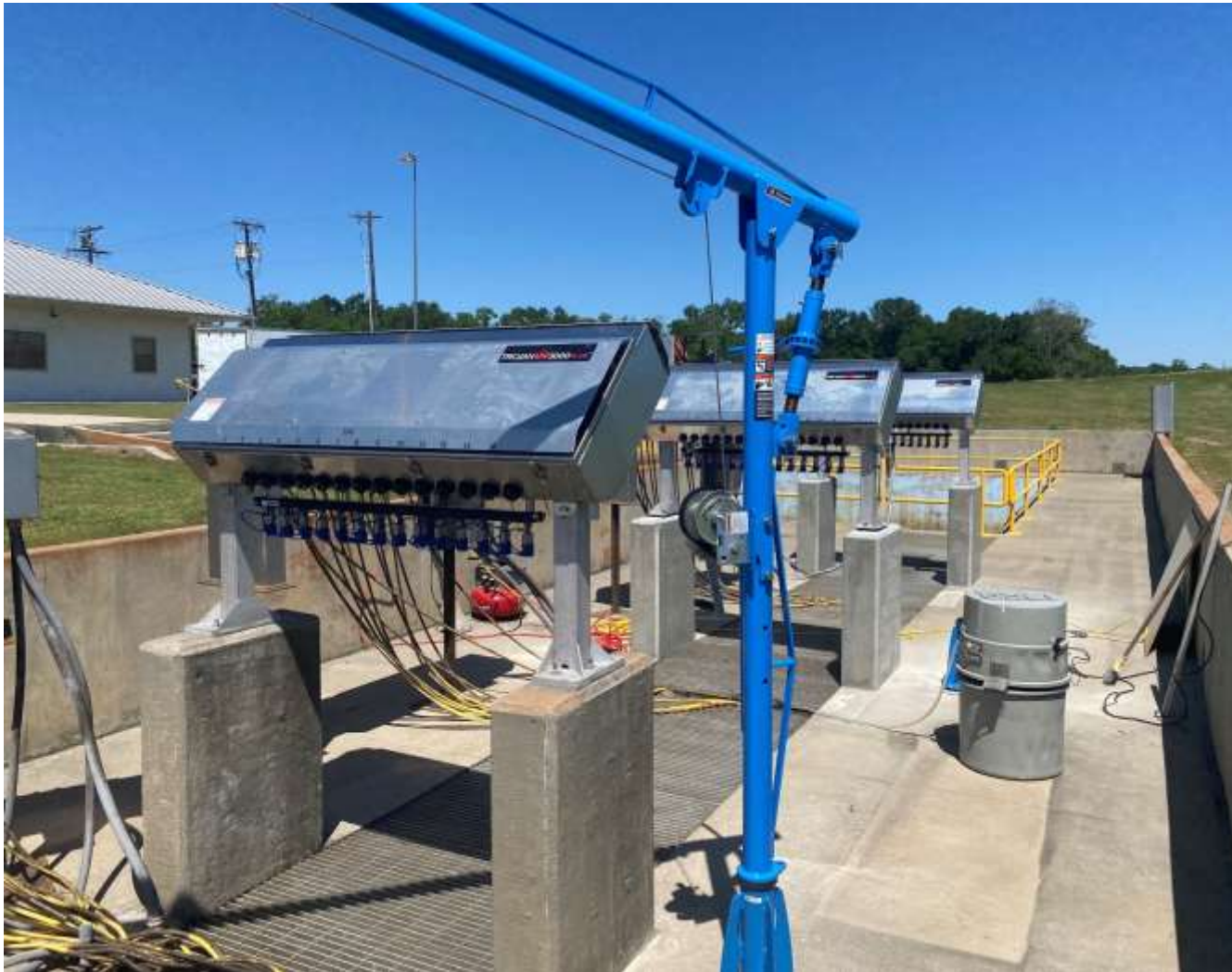
Picture 1 – New UV disinfection at WWTP
