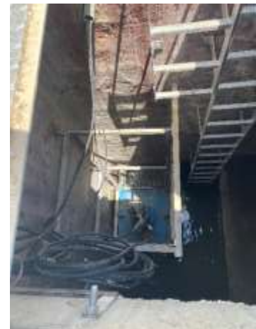
Picture 3: new comminutor at lift station
