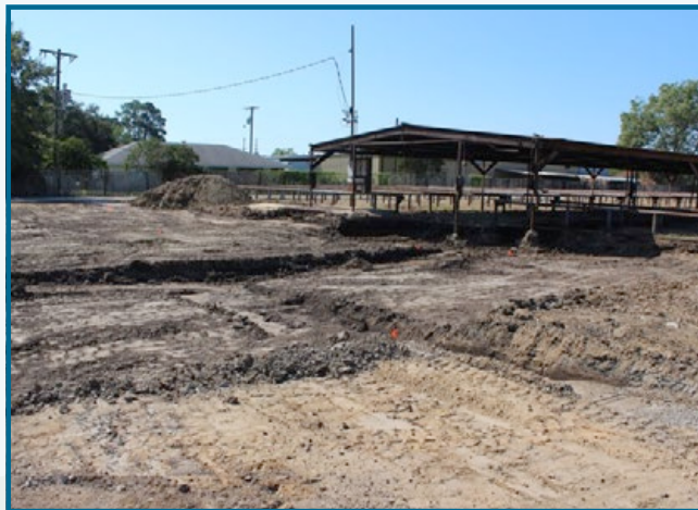
The nearly four acre site in Lafayette is undergoing soil sampling and removal of non-hazardous materials. Non-degraded dirt (from the pile in the background) will cover the area once soil tests show the site meets RECAP standards.
