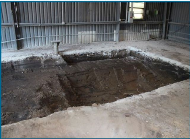
A sump from the interior of the main building has been removed, as the site undergoes excavation and sampling for constituents.
