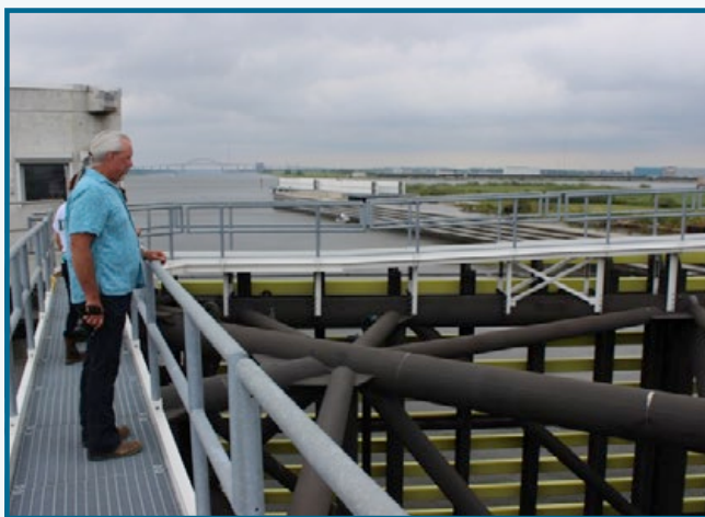
DEQ Geologist John Jennings examines the gate's hydraulic systems, which run on shore power through a 4-horsepower engine that typically applies between 900 to 1,000 PSI of pressure.
