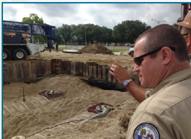
DEQ Environmental Scientist Laurence Carter observes the installation of three 20,000-gallon Underground Storage Tanks at a gas station in Baton Rouge
