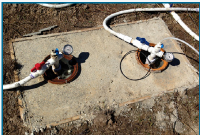
Several pump and injection well locations at the site are in place as part of the groundwater bioremediation process.
