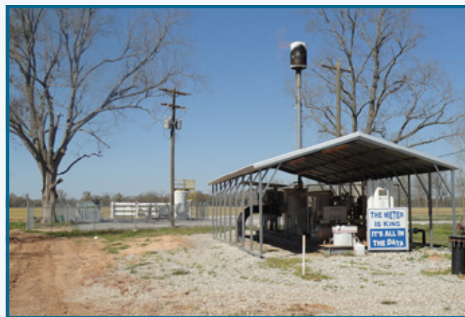
Gas Collection and CNG equipment
