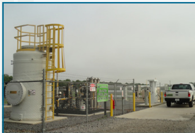
Parish truck fueling at the BioCNG fueling station
