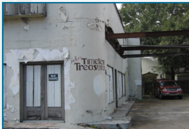
The Timeless Treasures site before remediation was a blighted property and an eyesore for the neighbors and the city of New Iberia.
