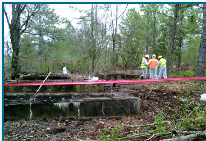
EPA contractors discuss the work in progress at the Ida Refinery cleanup in Ida.
