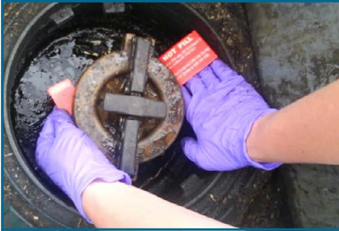
A red tag is placed on an underground storage tank to label the tank as noncompliant with regulations
