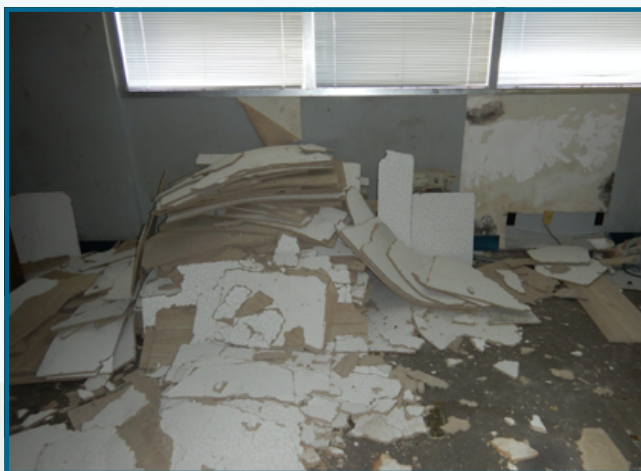
Interior photos from the federal building before remediation began.
