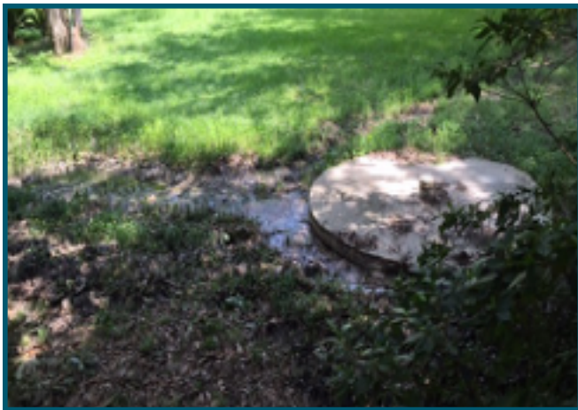
Figure 6. Sewage overflowing from an improperly managed home waste system
