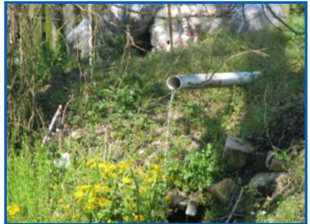
Discharge pipe from onsite sewage treatment system.
