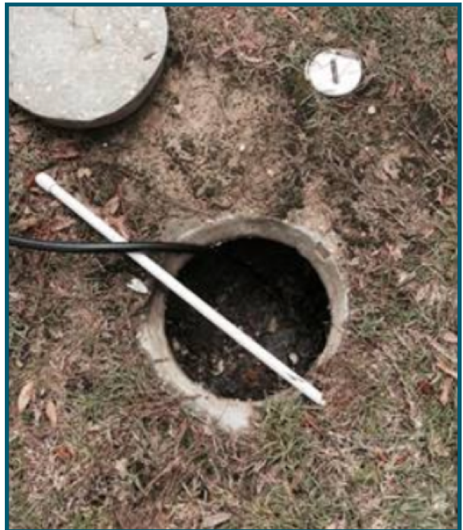
Figure 2. Home waste tank requiring pump out due to aerator not working for several years
