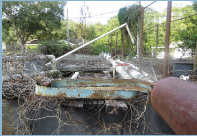
A poorly maintained sewage treatment plant operated by Savoy.
