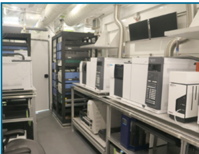
State-of-the-art equipment in the MAMLs will be a benefit to the air monitoring process.
