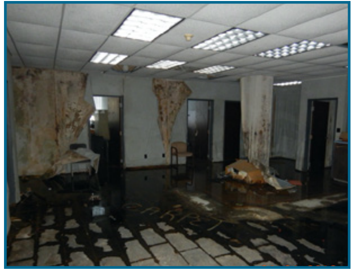
Interior photos from the federal building before remediation was started.
