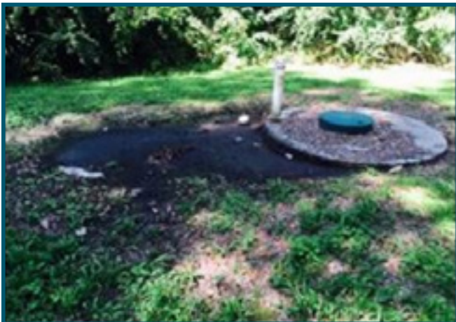
Figure 5. Sewage overflowing from an improperly managed home waste system
